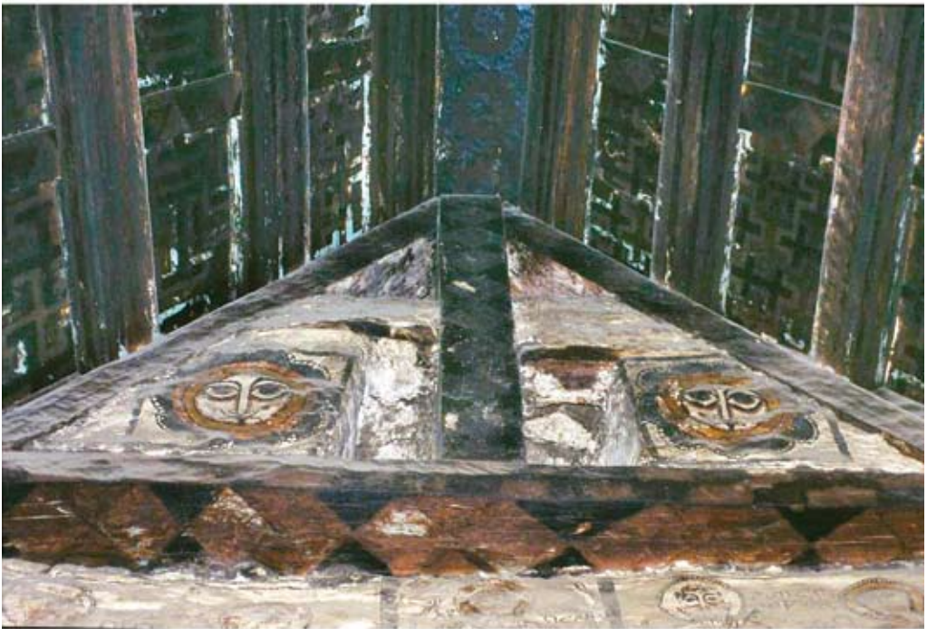
14. Ēmäkina Mādḡane Aläm church, gables at east and west ends of the nave
