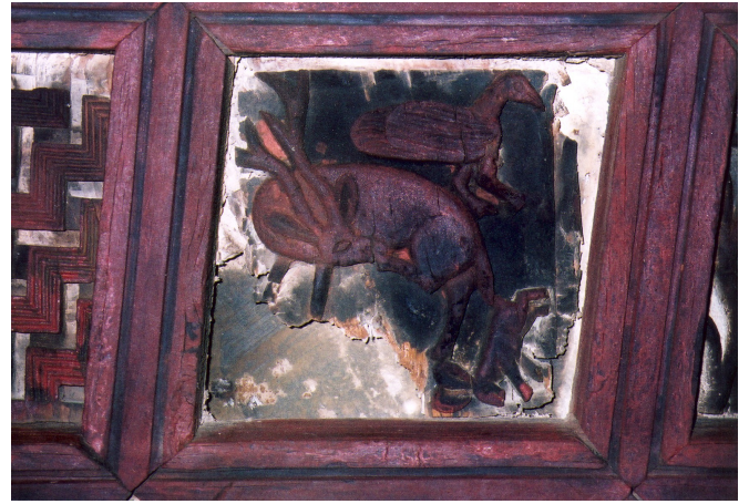
Detail: One of the reliefs which is decaying.
