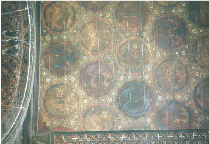
Ceiling damaged by smoke with hardly visible decorative painting.
