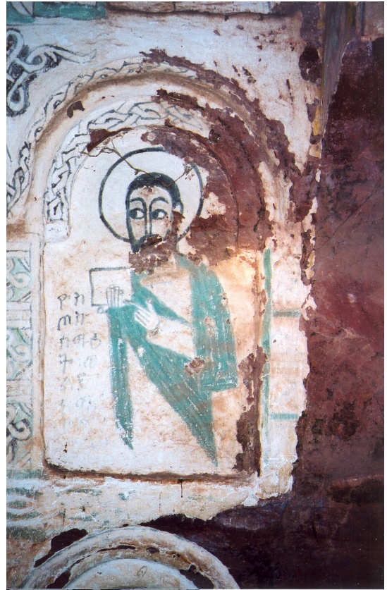
Detail: The plaster has started to fall, in the long run nothing will be left.
