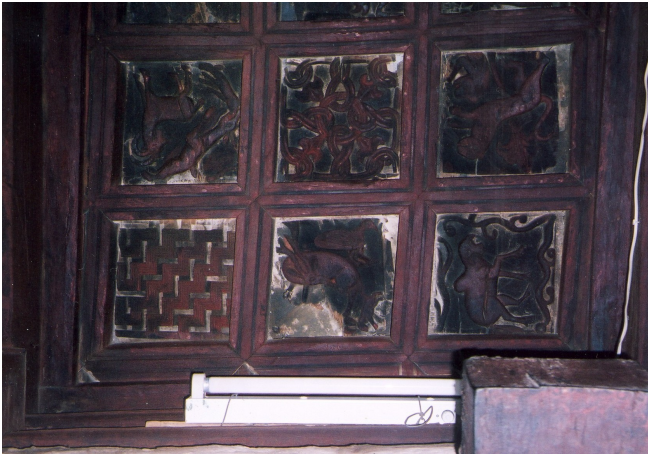
The wooden ceiling in the narthex. The reliefs are drying out and falling down.
